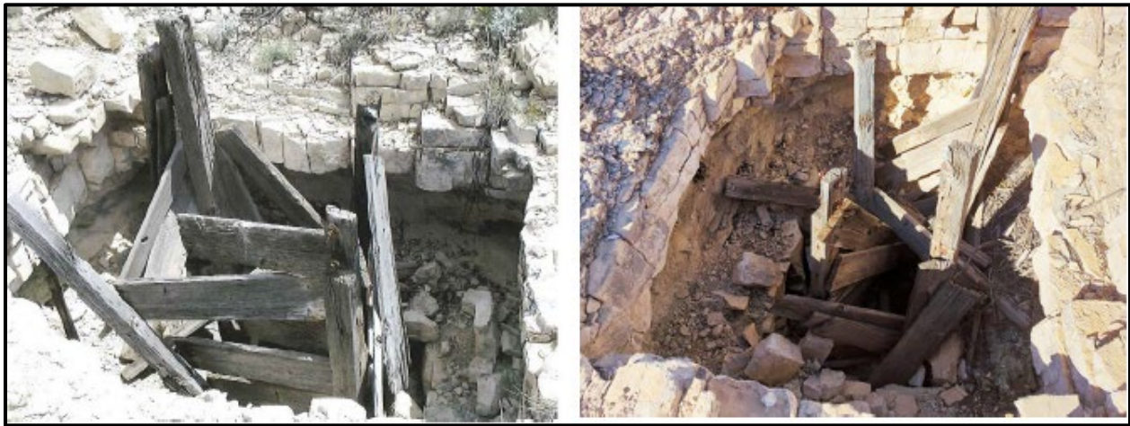
Figure 3.) Feature 1 at LA 182556, Mine Shaft Collar Timber Shoring 2015 vs. 2023 (Kibler and Kurota 2024, NMCRIS 154823)
