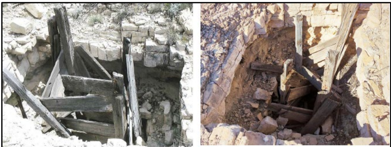
Figure 3.) Feature 1 at LA 182556, Mine Shaft Collar Timber Shoring 2015 vs. 2023 (Kibler and Kurota 2024, NMCRIS 154823)
