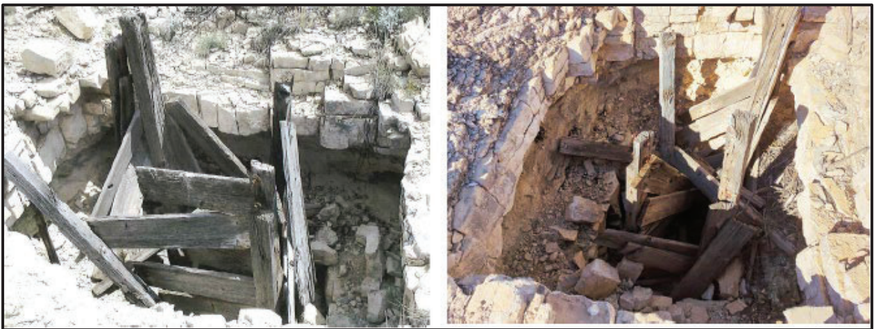
Figure 3.) Feature 1 at LA 182556, Mine Shaft Collar Timber Shoring 2015 vs. 2023 (Kibler and Kurota 2024, NMCRIS 154823)
