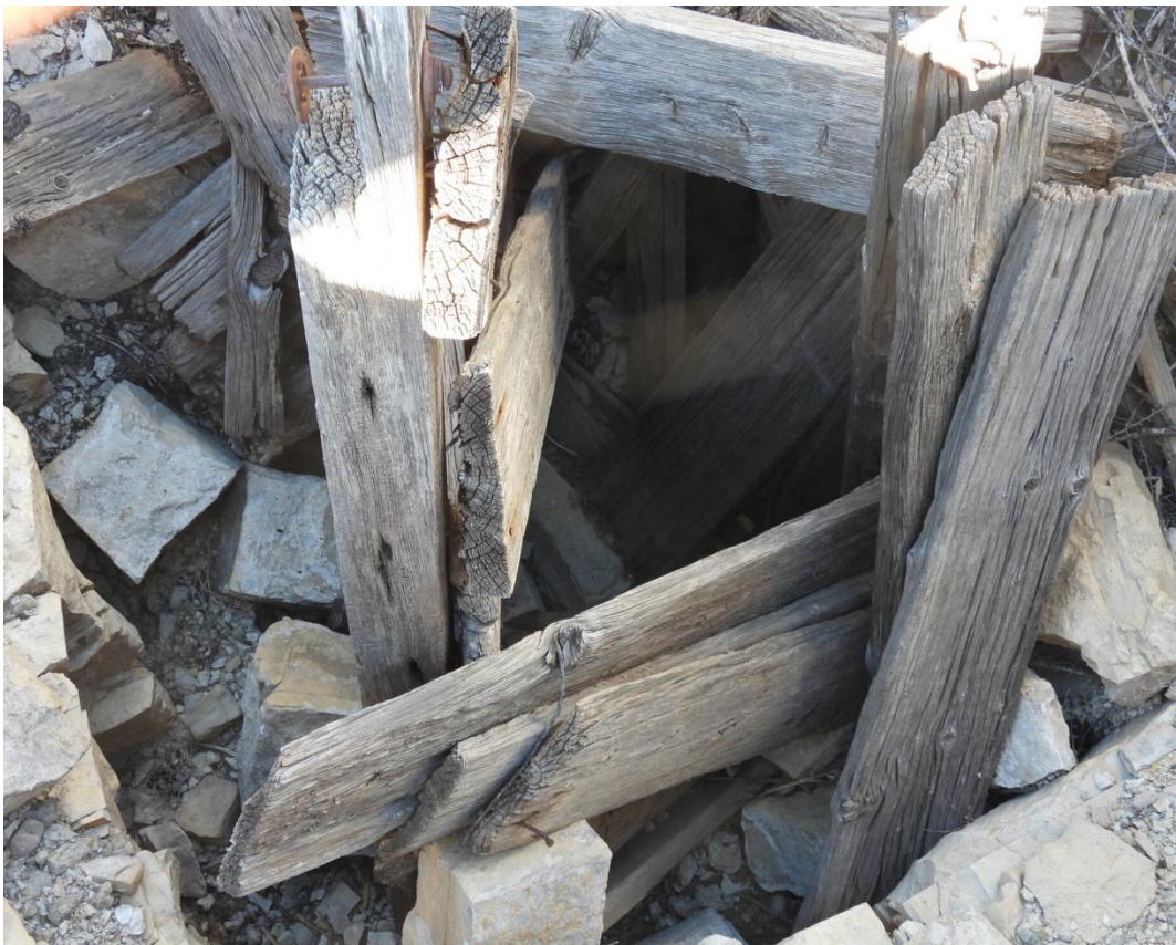
Lone Eagle Shaft BLM: The collar is obstructed by collapsed timbers and provides no flyway. BCI Photo by Jackson Bain
