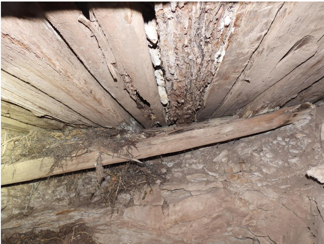
Lone Eagle Root Cellar: Ceiling of the feature could easily collapse under load. BCI Photo by Jackson Bain
