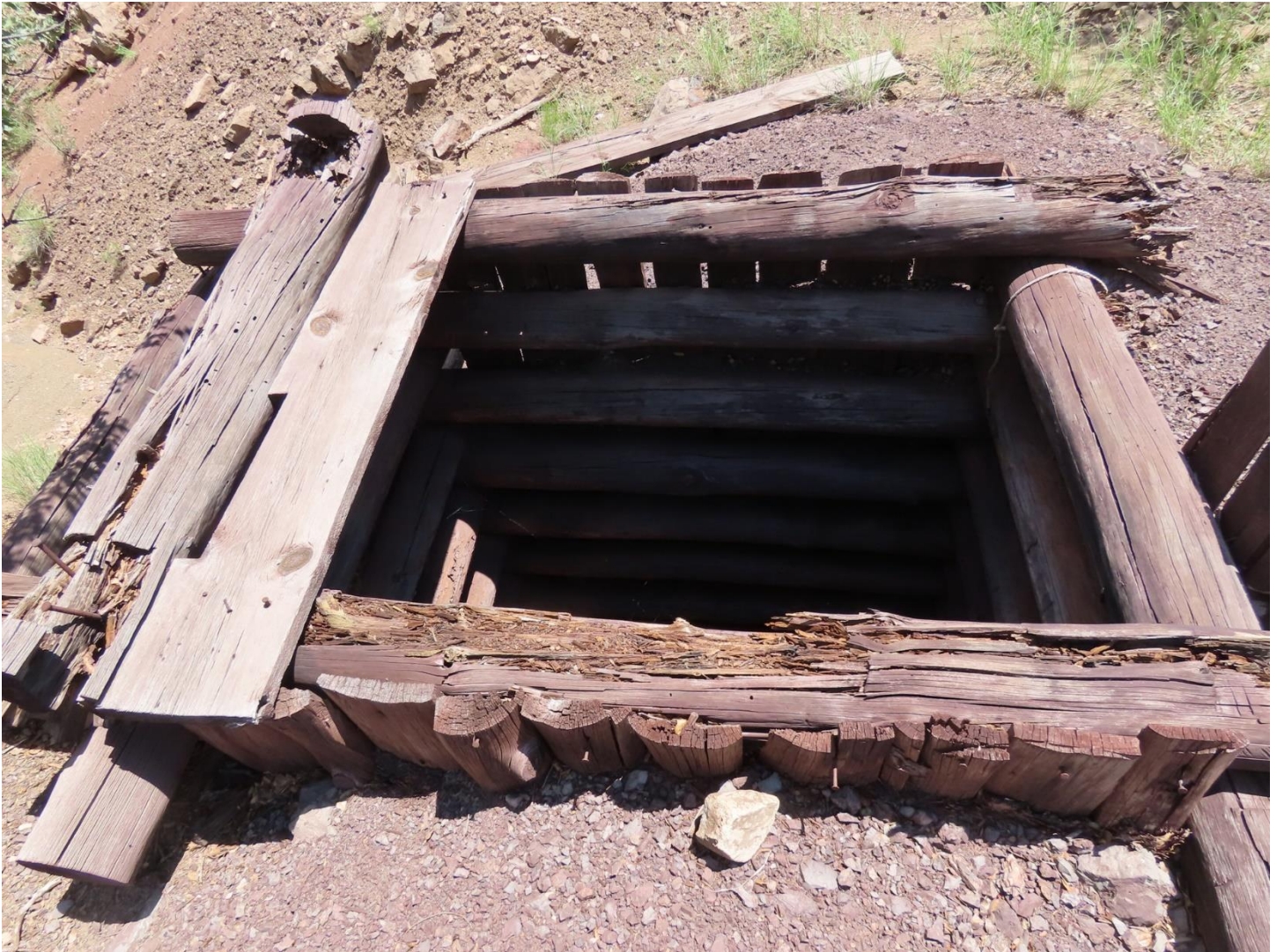
Homick Energy Maggie Mine Shaft: Sturdy timbers support the collar of this mine shaft. BCI Photo by Dillon Metcalfe
