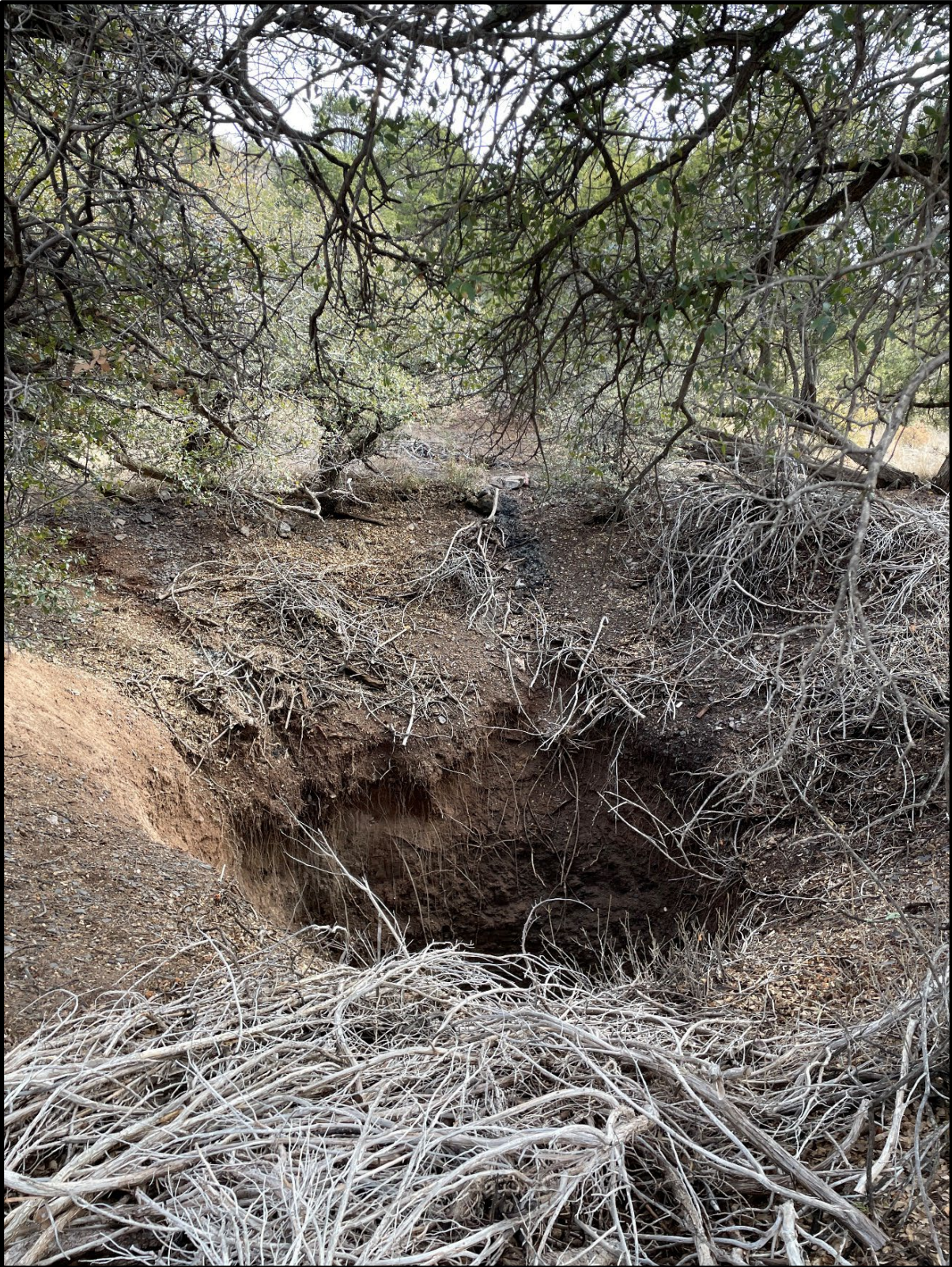
Figure 1. Subsidence Feature Field Photo
