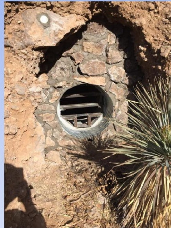
Rock bulk-headed culvert with bat-friendly gate. Cemented rocks assist with blending into landscape
