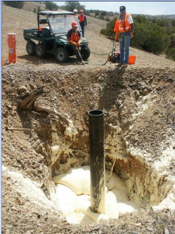
Polyurethane foam plug with a drain pipe (Cerrillos Hills State Park)
