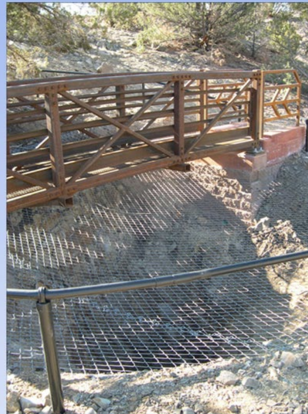
The completed mesh and bridge installation over a shaft (Cerrillos Hills State Park)
