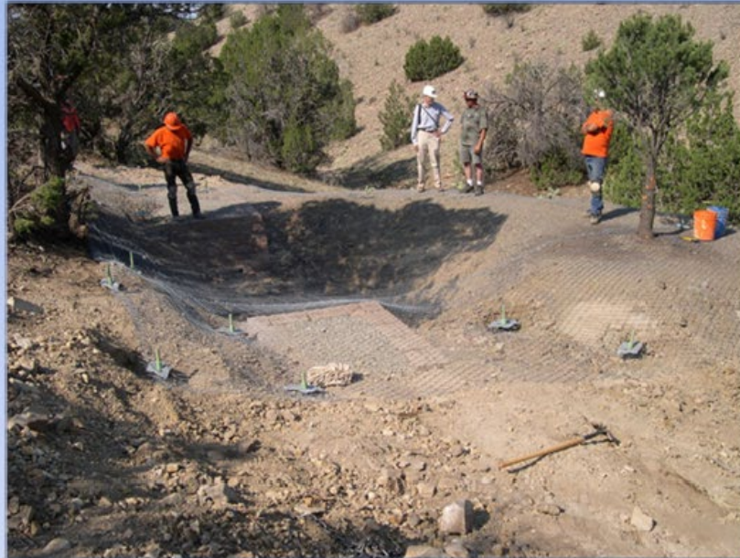
Installation of high-strength steel mesh with rock anchors. Note the partially completed bridge abutments on two sides of the shaft opening.
