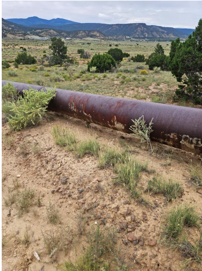
Unknown Material on Pipe
