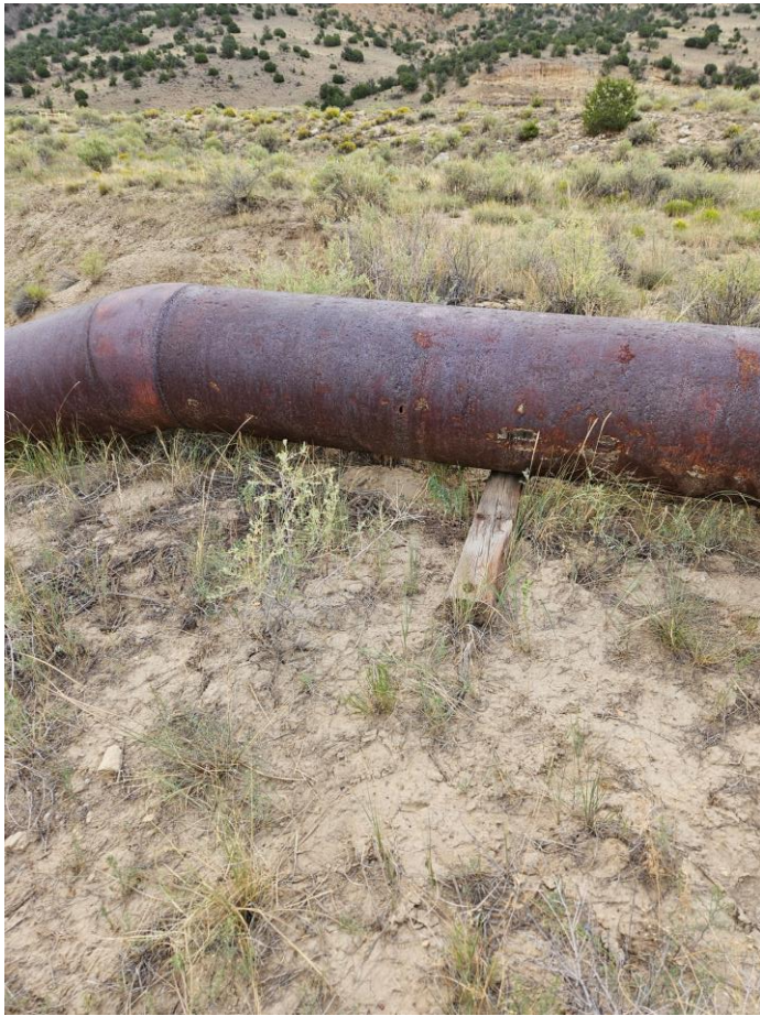
Bend Near Point of Discharge
