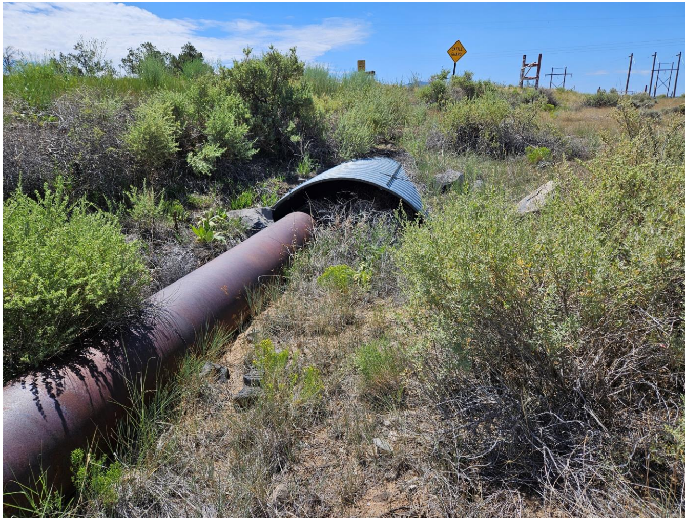
Pipe in CMP Crossing with Heavy Sediment Fill
