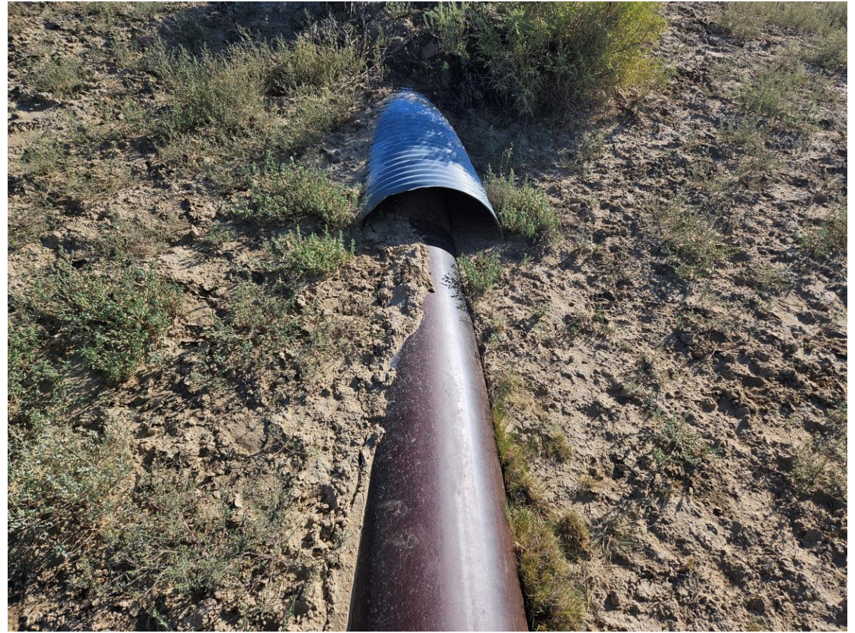
Partially Buried Pipe in CMP Crossing
