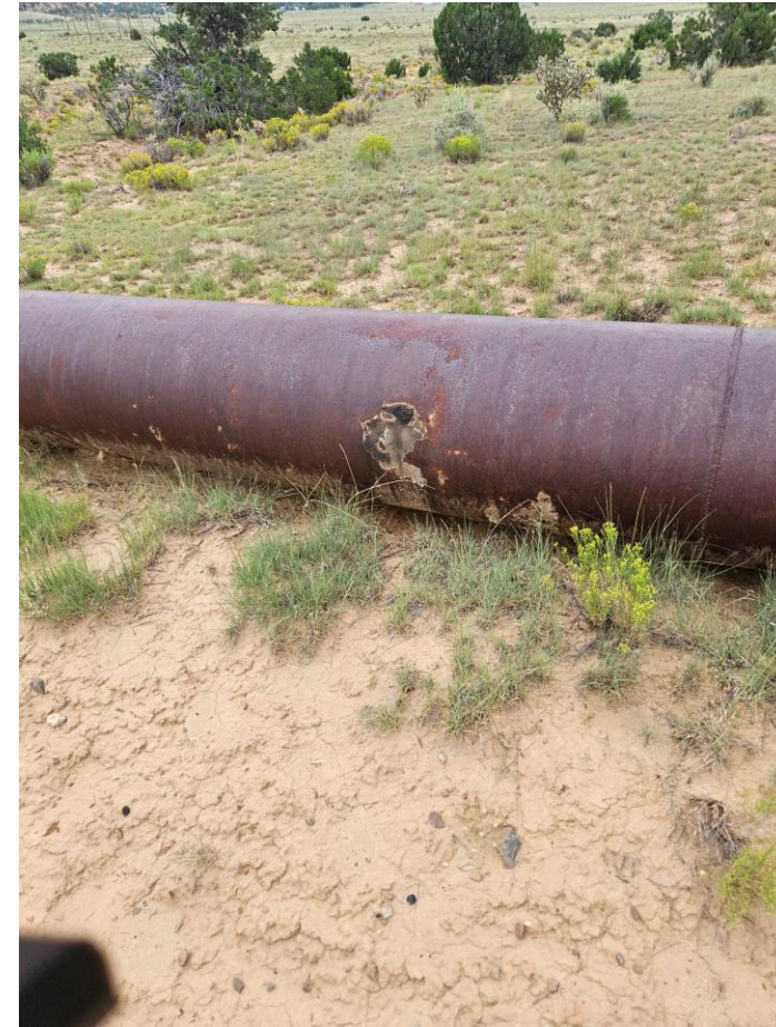
Unknown Material on Pipe
