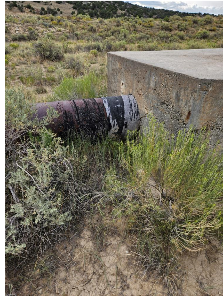
Unknown Material on Pipe and Thrust Block Interface
