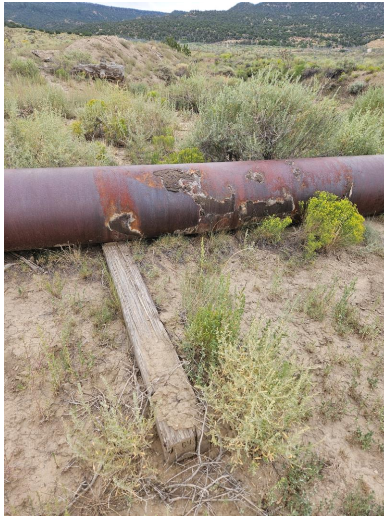
Unknown Material on Pipe
