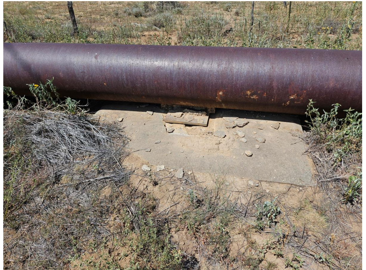
Broken Bolts with Steel Plate Welded into Pipe and Bolted in Concrete
