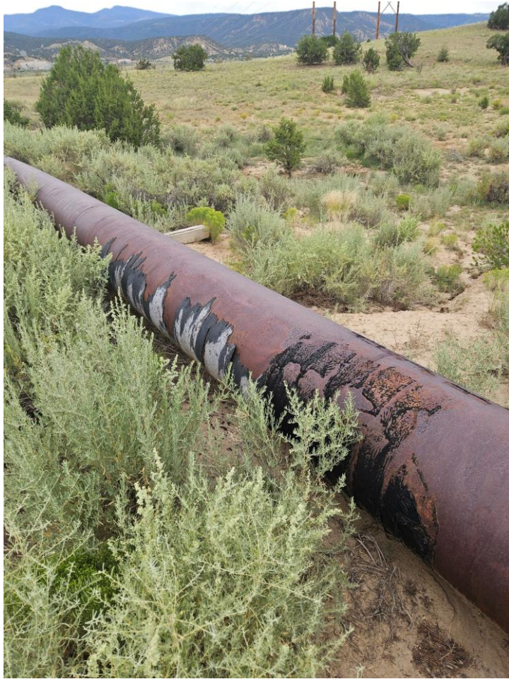
Unknown Material on Pipe
